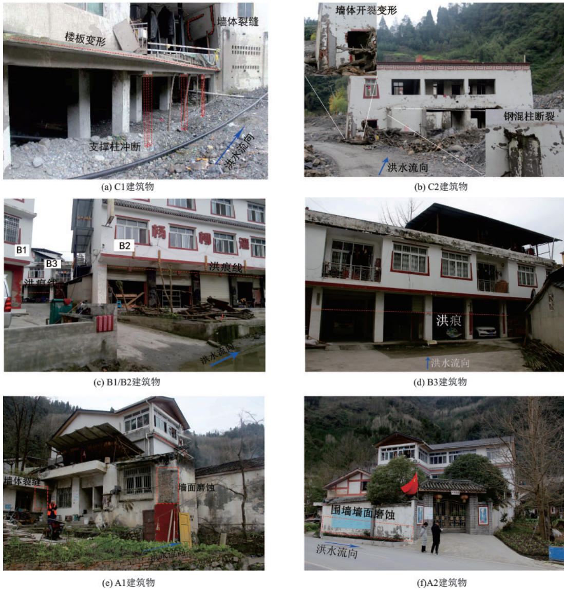
图4 建筑受损破坏情况 Fig.4 Damage of buildings
